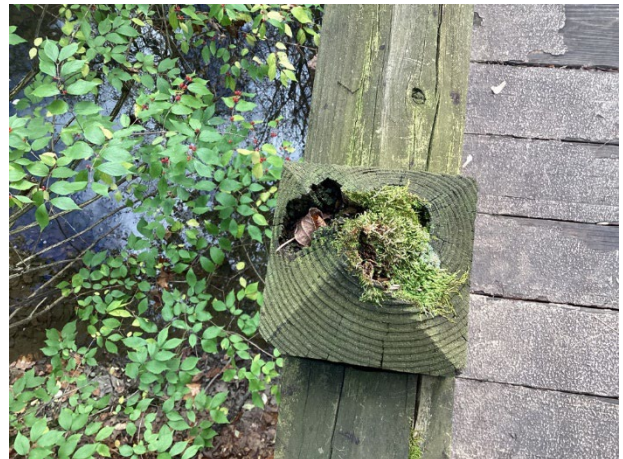
Wood rot and organic growth
