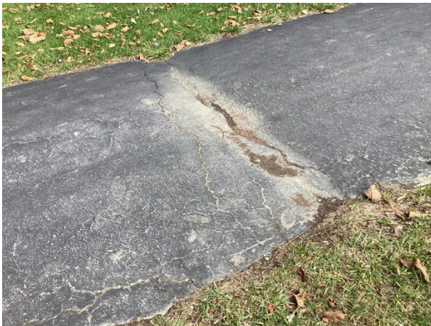
Evidence of standing water
