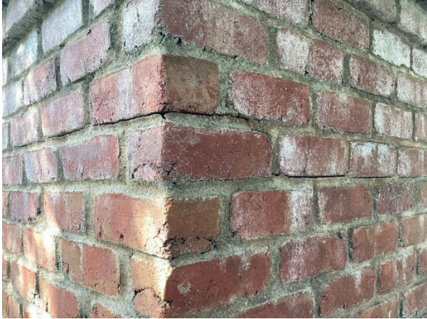
Mortar cracks and deterioration at Bishops Wood Rd
