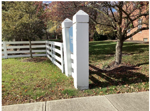
Leaning post at Mead Way
