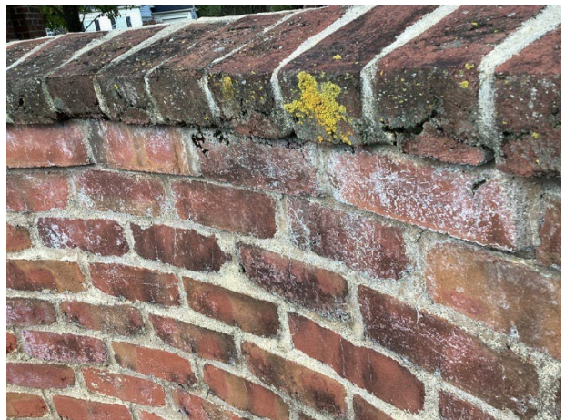
Masonry deterioration at Brooksvie Dr
