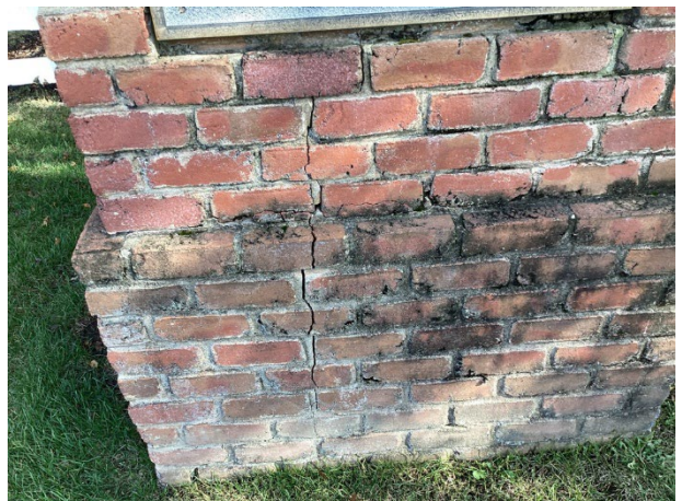
Masonry cracks and organic growth at Bishops Wood Rd
