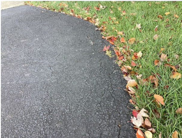
Settlement cracks (Annabelles Green)
