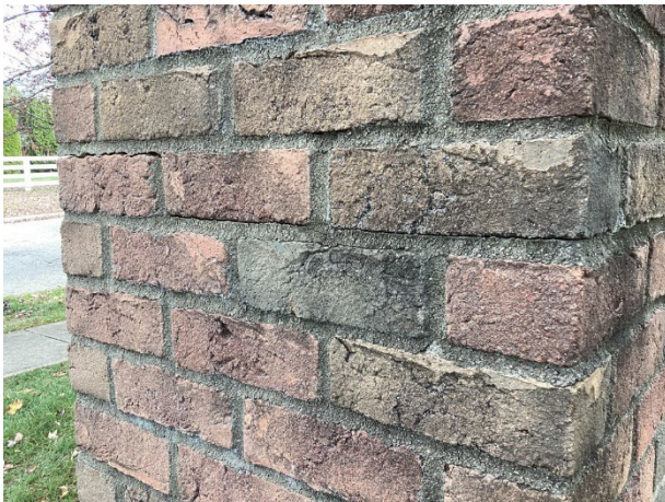
Mortar loss at Abbotsbury Ct
