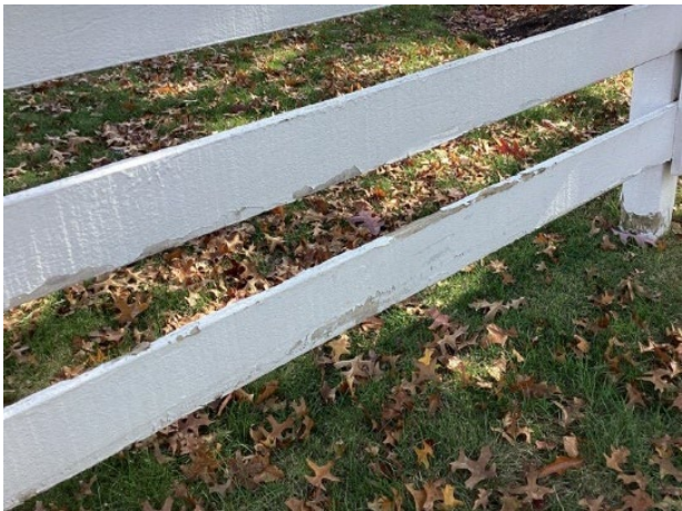
Periodic peeling finishes
