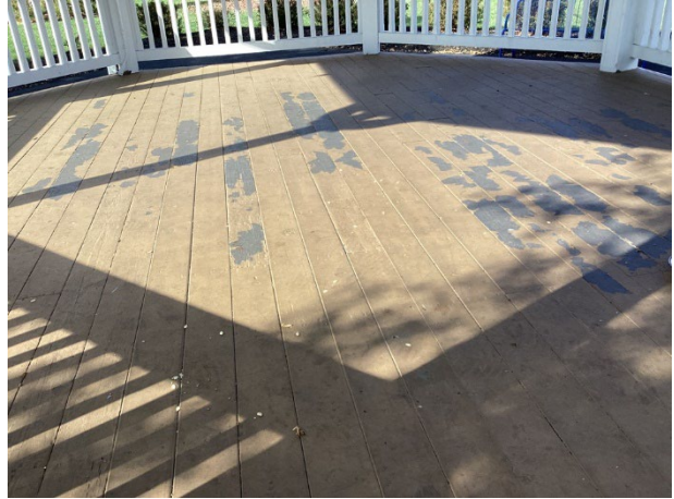
Finish deterioration at deck boards
