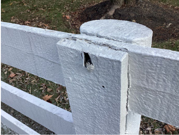
Wood rot at recently stained fence, shown at Heath Gate Drive
