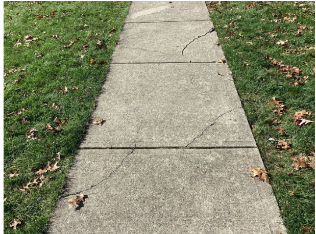
Sidewalk cracks and damage
