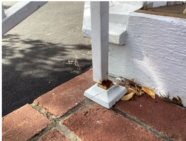
Detached railing and rust
