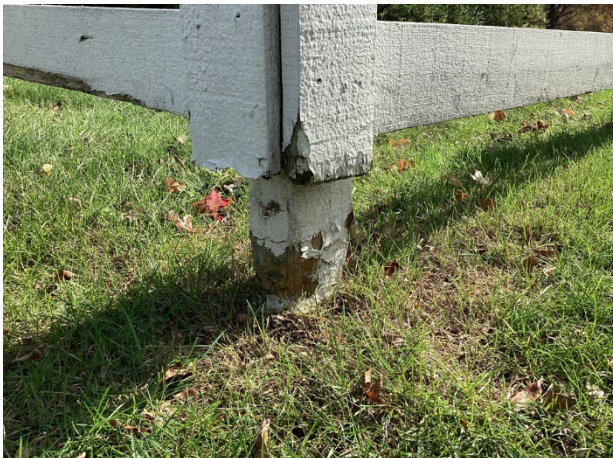
Wood rot and landscaping damage
