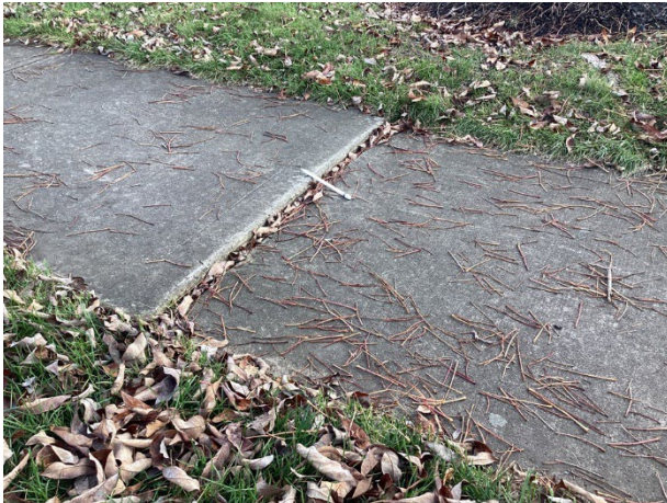
Isolated trip hazards
